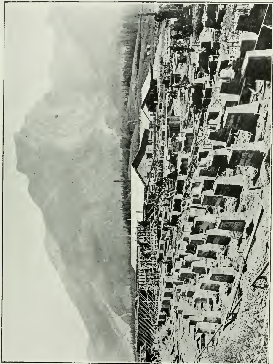
Western Canada Cement and Coal Co., near Banff. The largest plant in the Dominion under construction. Capacity 2,000 bbls. per day.
